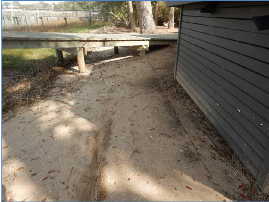
Photograph 5: Visible Impacts to Rear Deck
